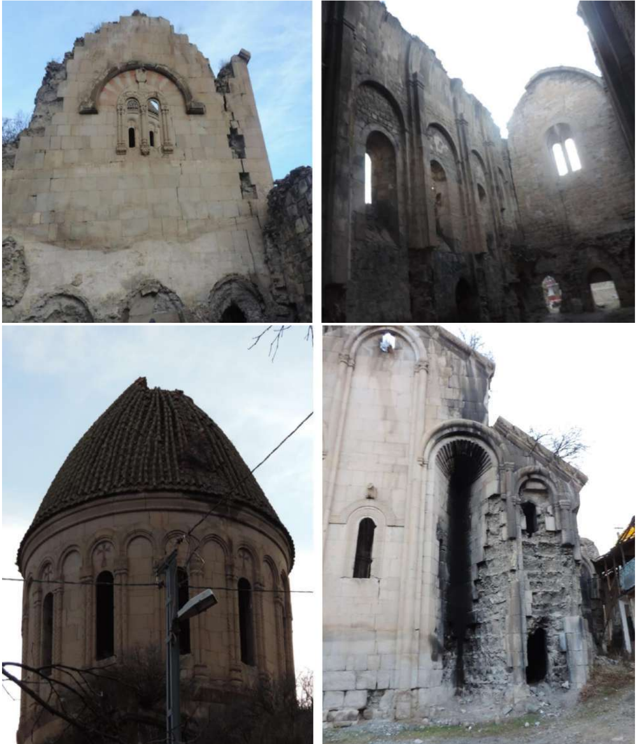
Figure 3. Some Structural Damages of Erzurum Oshki Church
