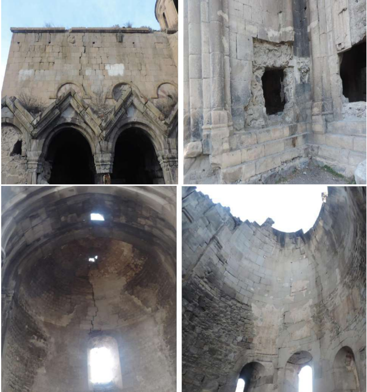
Figure 4. Damaged Dome and Apse Section on the Interior Facade of the Structure
