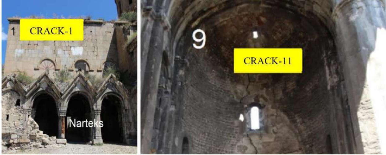
Figure 7. Location of the Crackmeters (Device 1 and Device 11)
