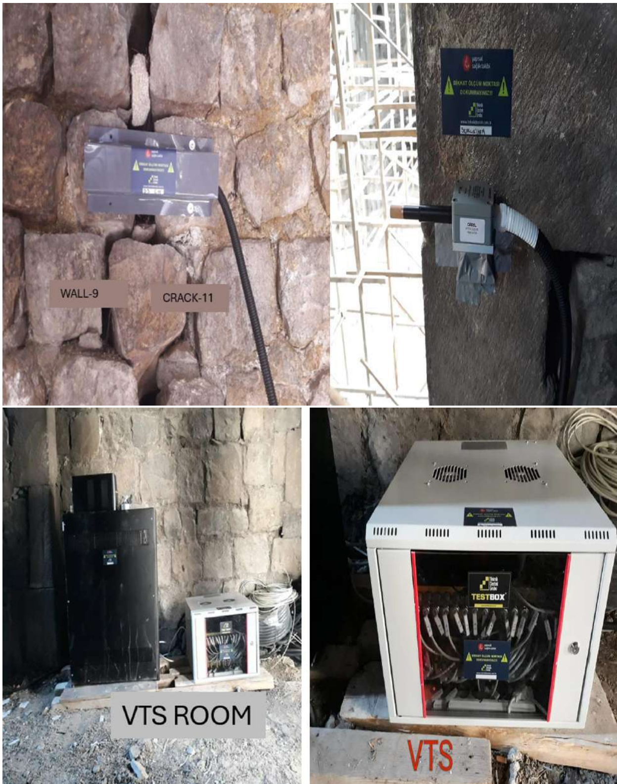
Figure 5: Some devices of SHM Equipment
