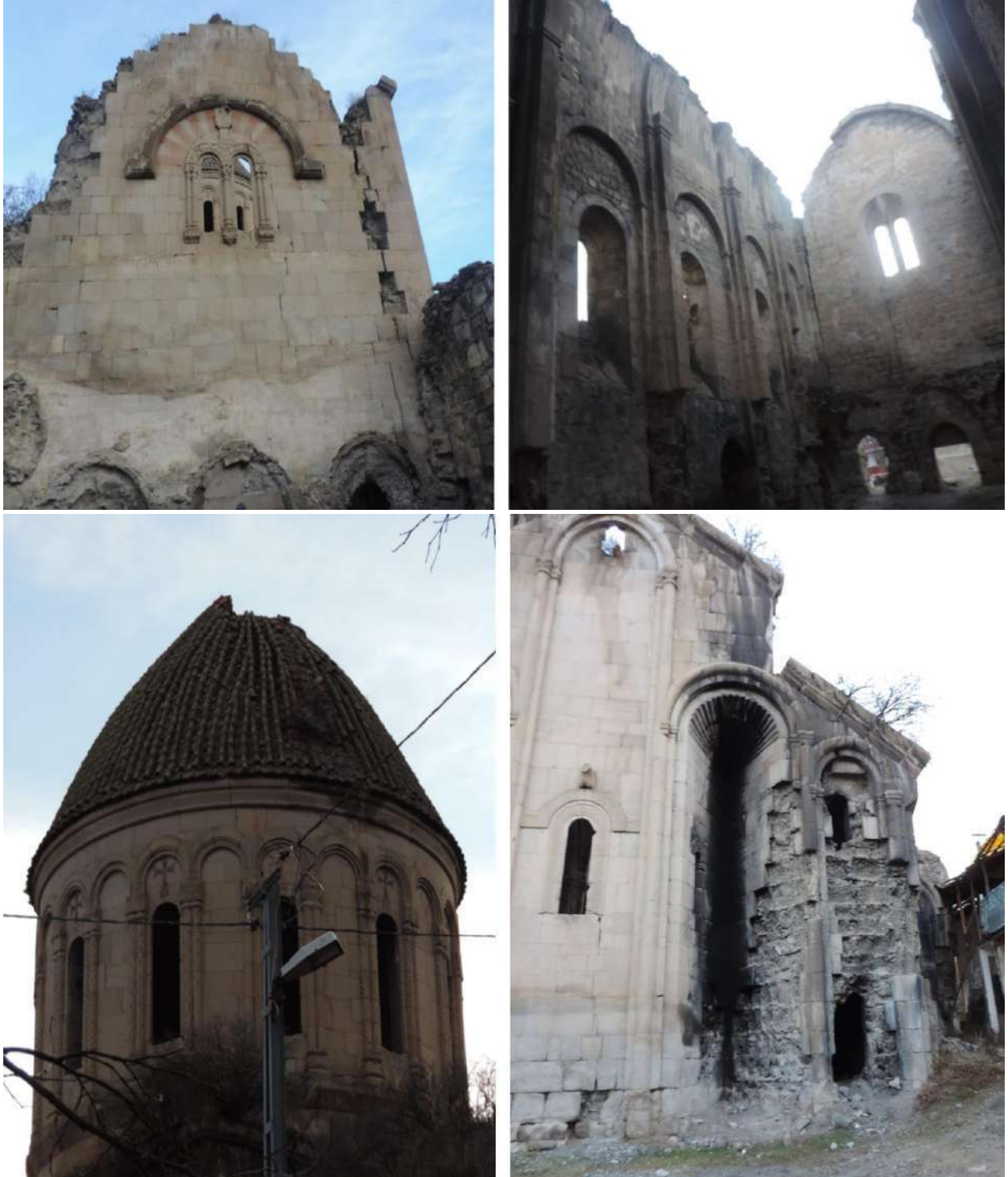
Figure 3. Some Structural Damages of Erzurum Oshki Church
