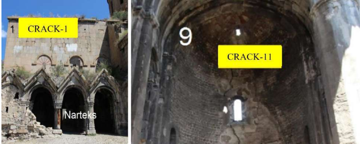
Figure 7. Location of the Crackmeters (Device 1 and Device 11)
