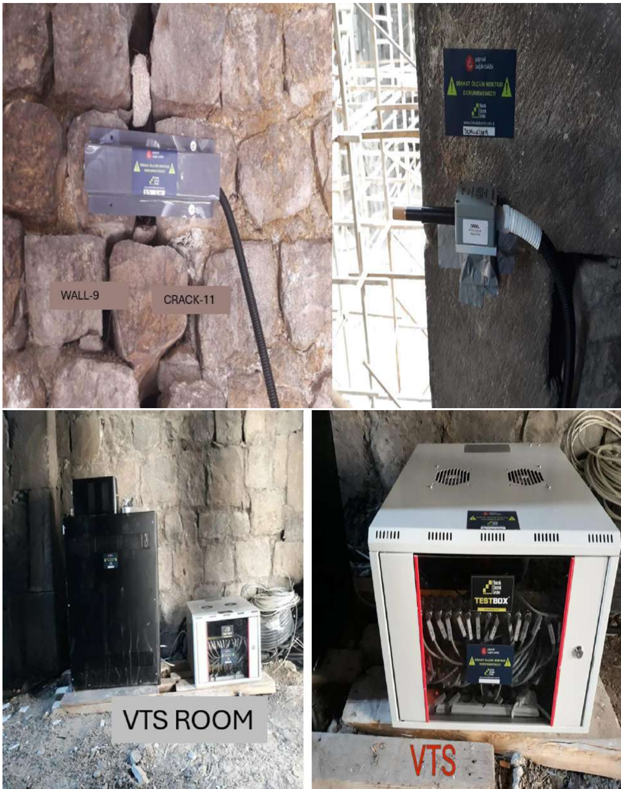
Figure 5: Some devices of SHM Equipment
